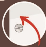
Toilet stall: area around locking mechanisms
