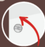
Toilet stall: area around locking mechanisms
